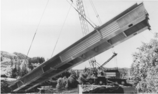
Fig. 26 The Foresmo Bridge in northern Norway is an excellent example of the use of aluminum-magnesium alloys for built-up girders systems; this photograph illustrates a major advantage of replacement aluminum bridges—the ability to prefabricate the spans and move them in place quickly, minimizing the disruption to traffic.
